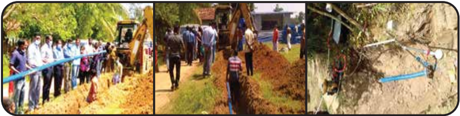
Pipes were laid in Kothiyapula in order to supply clean water to the school in the area. The water pressure was also checked to ensure a stable supply of water
